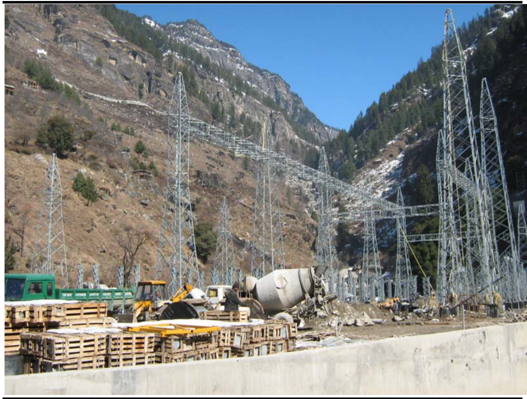
Figure 1.1 Switchyard at Prini
